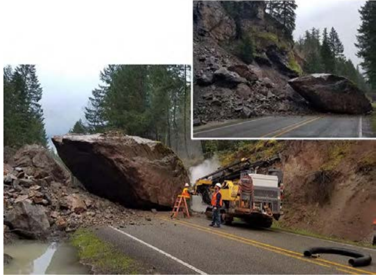
Rockfall in Oregon, USA. Source: Oregon DOT
